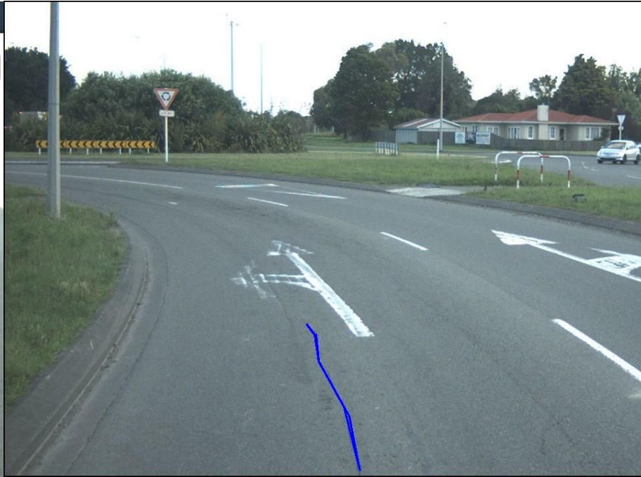
Linear length of a longitudinal crack can also be estimated using correct calibration factors. This one is about 6m.
