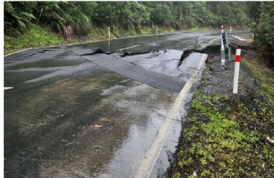
Road damage has contributed to the proposed increase, the council says. Photo: RNZ
