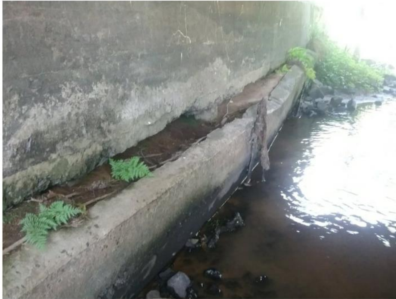
Scour (Element 29): Failure of abutment B protection structure.
