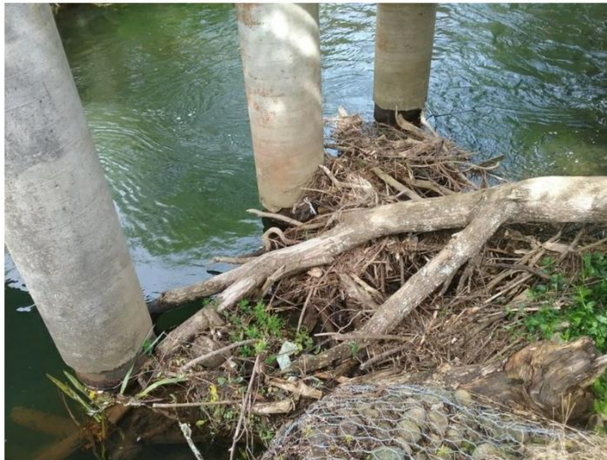
Invert / River Bed (Element 25): Log jam impeding flow at A.
