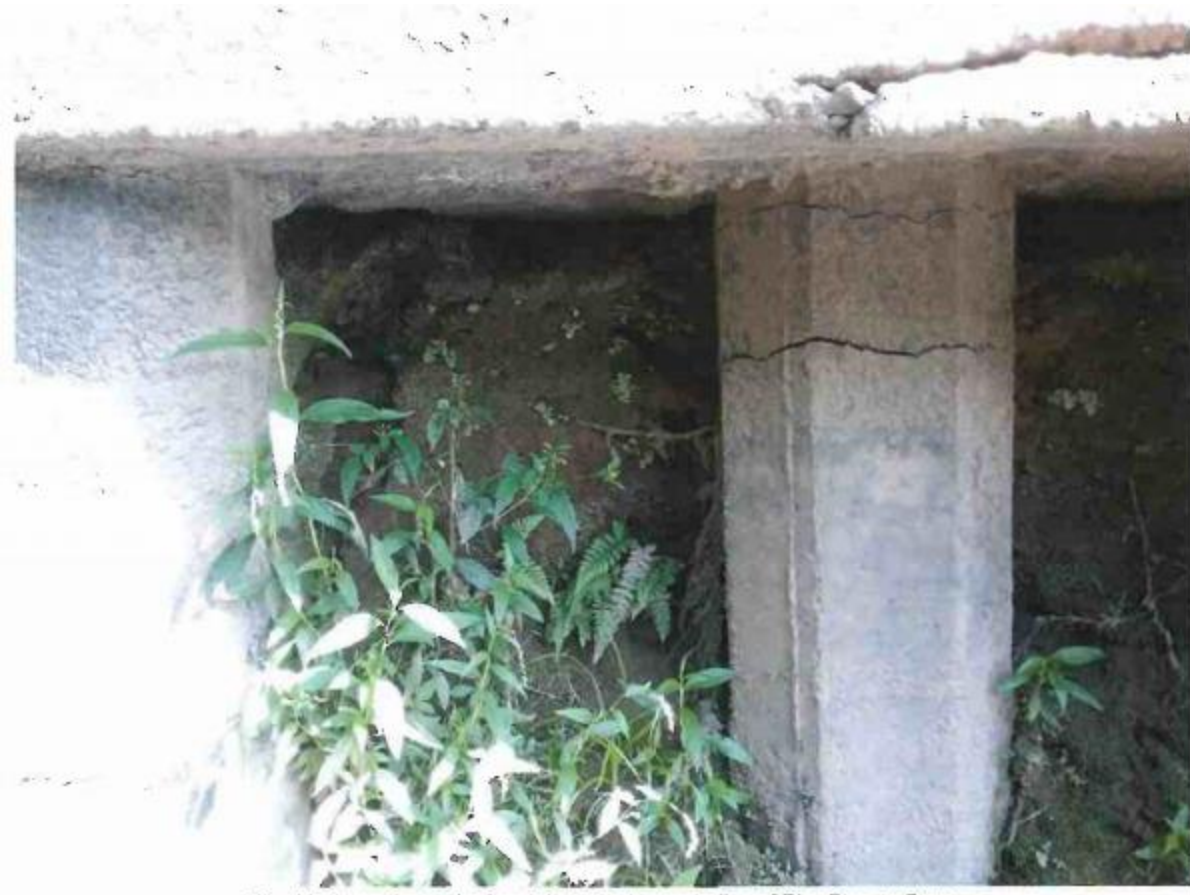
Pier / Column: Large horizontal cracks to most piles of Pier D up to 5mm.
